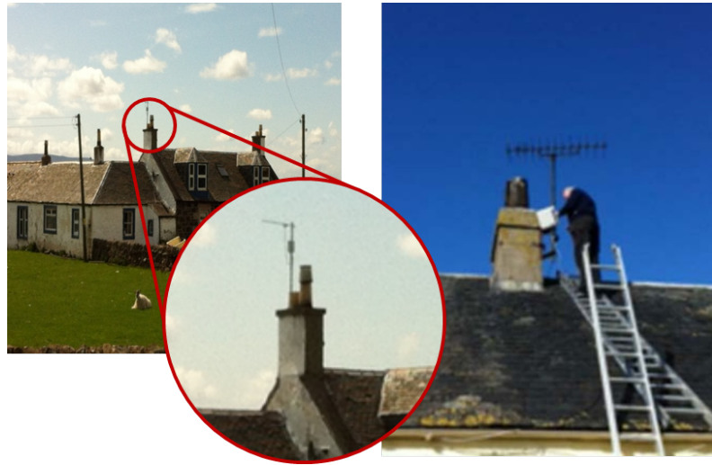
Figure 9.3: CPE installations at trialists' premises.
