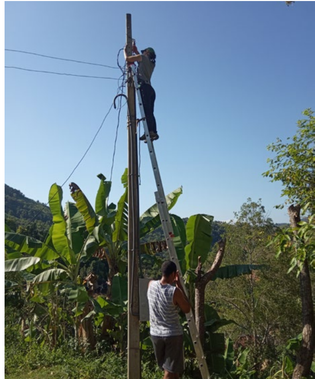
Setting up a community network node at the top of a power pole in the quilombo Ribeirão Grande/Terra Seca.
